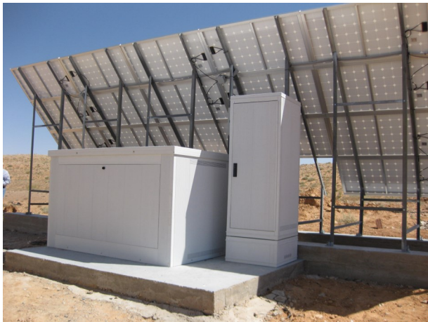
Above view of a BATT'BOX with an outdoor cabinet on site
